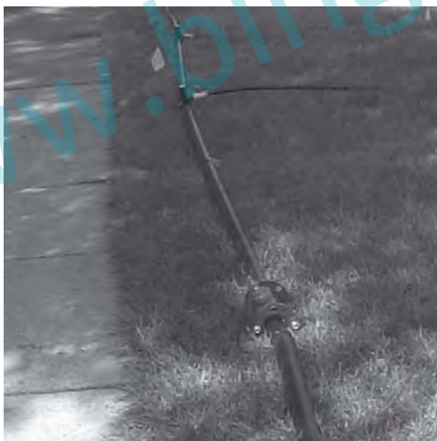
Figure 19 Example of Above Ground PE Bypass Pipe
