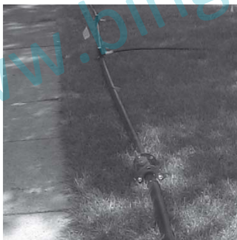
Figure 19 Example of Above Ground PE Bypass Pipe
